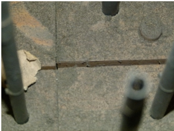
General level of dust & dirt
